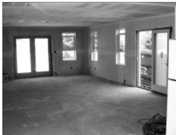
A concrete floor was poured underneath the 40x40 addition, allowing for a crawl space. The new room is built off the existing kitchen for a welcoming gathering space.
