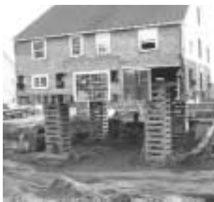
The building was held up on cribbing while Mark replaced rotten beams and installed new posts.
