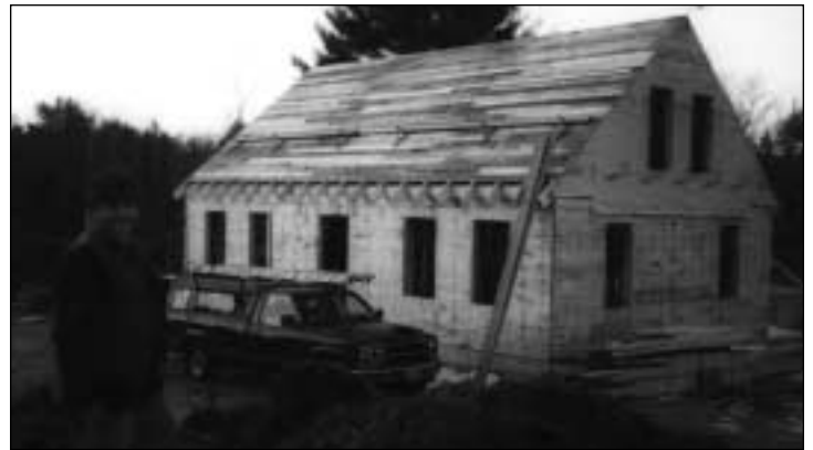
Above: Wide sheathing was used for the exterior walls. Below: Narrow sheathing from a woodpile placed close to the home is used to complete the roof.
