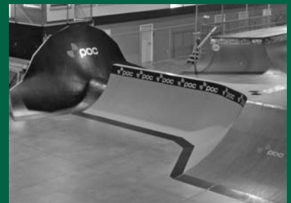
Rye Airfield's new Hip-Spine-Roller ramp was built with materials from Rand Lumber.
