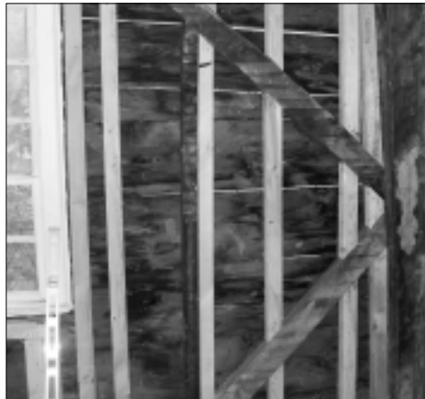
Sistered studs: Cured hemlock studs are sistered with the existing wall supports.
