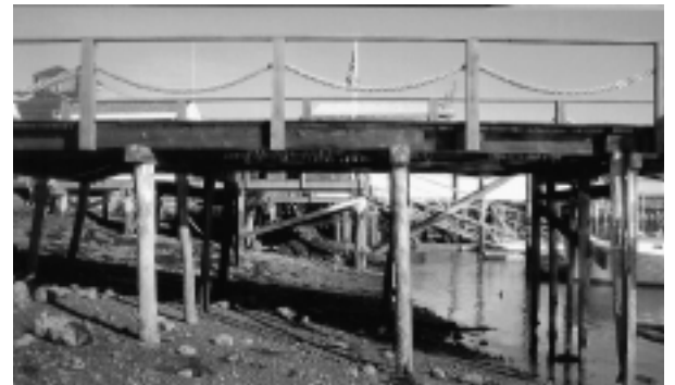
Photo of old piles/pier, ready to fall apart
