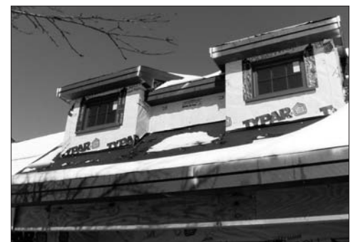
Rand provided rough sawn lumber for outside details such as the two dormers on the front of the house.
