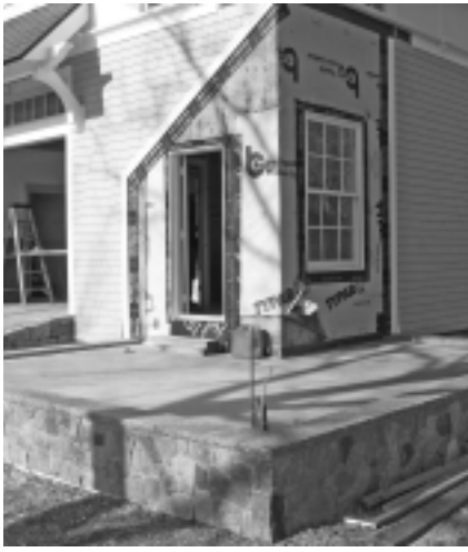
A greenhouse will be built off the side of the barn. A radiant heating system is built into the concrete slab.
