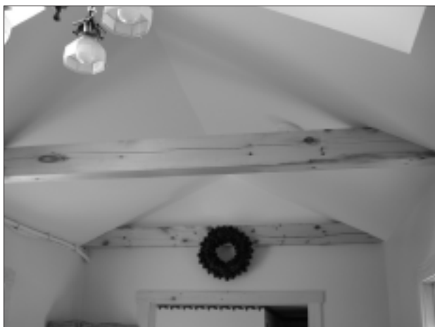
The four-inch by six-inch exposed beams with collar ties used in the connector section were custom-milled for the Walker home.
